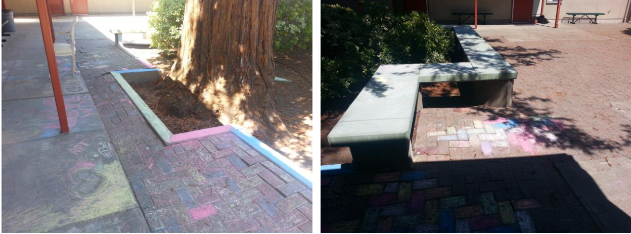
Walkways and hardscape areas require smoother surfaces to reduce trip hazards.
