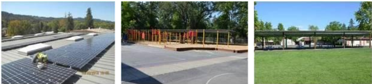
Solar panel installations on the newly constructed high school gym (left) and at the elementary school (middle, right).
